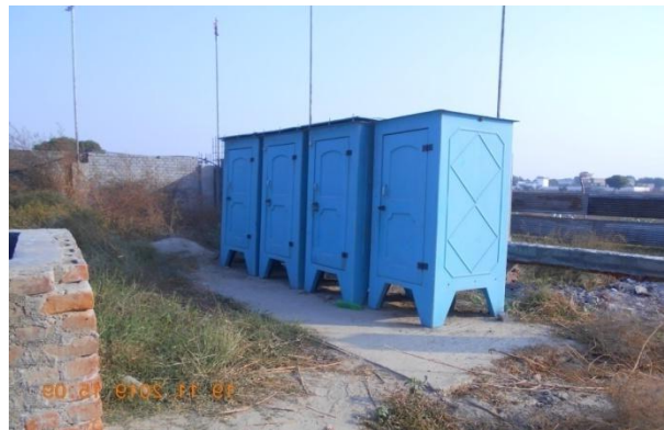
Figure 2.3- Temporary Toilet Facility at site
